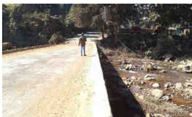
No delineation or edge protection on the causeway, Km 24+000
