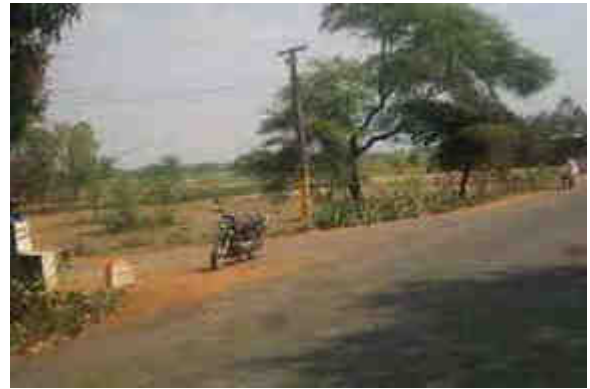
Absence of road marking at Km 35+300
