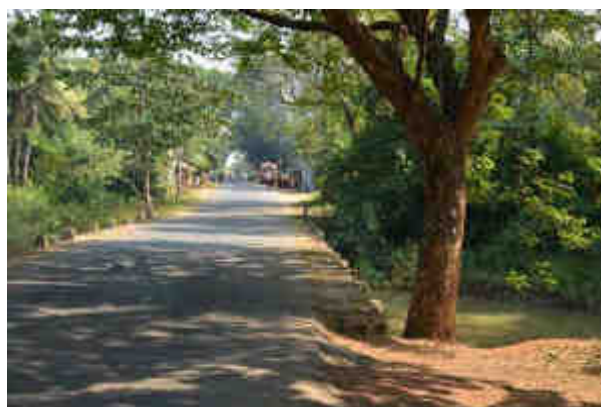
Absence of Parapet wall at Km 41+150
