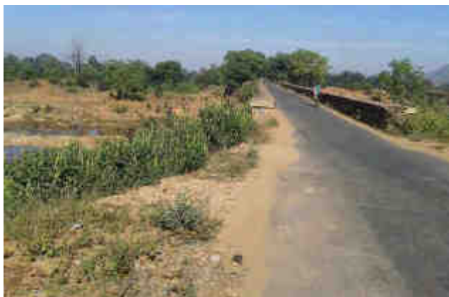
Bridge at Km 313+300, no edge protection on approaches
