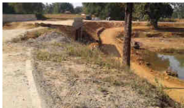
Sharp curve on high embankment without edge protection near approaching culvert (under construction), Km 31+800
