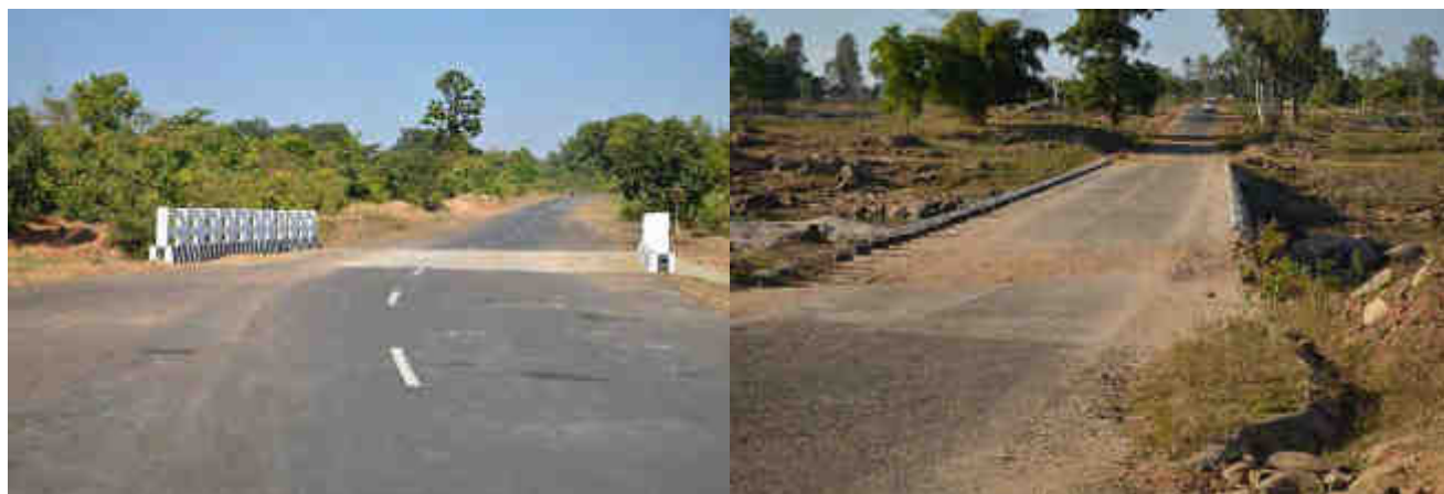
Absence of OHM on structure at Km 44+500 and submersible structure at Km 58+900
