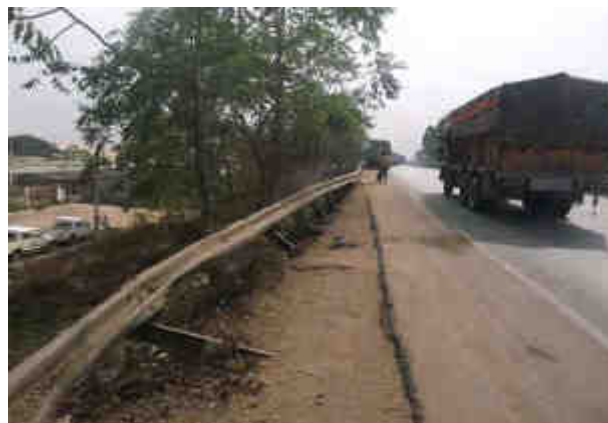
Broken crash barrier at Km 250+300
