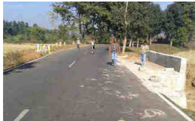
Unprotected approach to culvert under construction – lack of warning signs and barricades, Km 9+200
