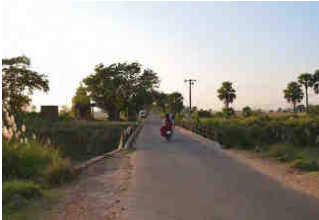
Missing bridge approach protection at Km 9+600
