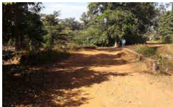
Parapets broken on culvert at Km 11+200
