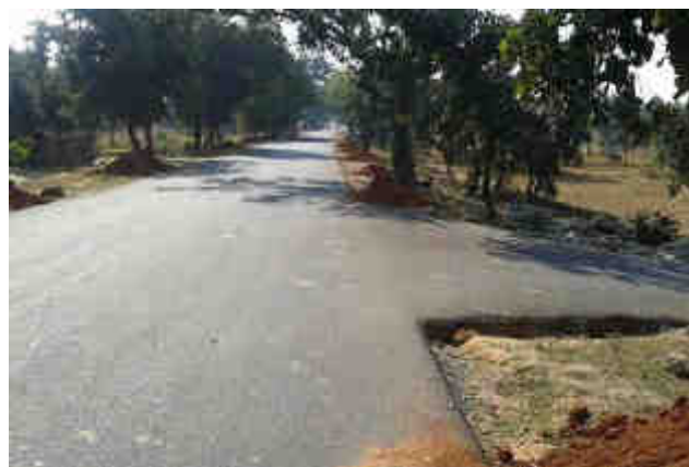
Side road joining with steep gradient, Km 9+000
