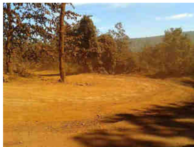
Hairpin bend with poor road condition at Km 11+400
