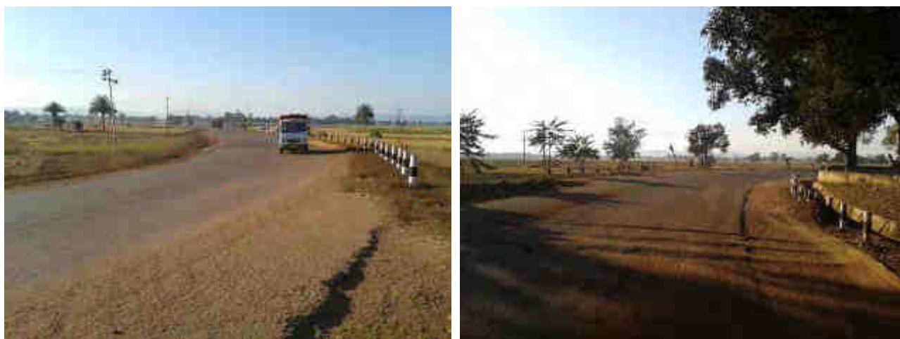
Lack of delineation in the stretch of road from Km 45+000 to 43+000
