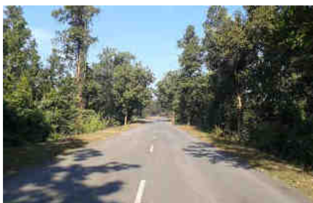
Lack of edge line in the stretch from Km 4+000 to 5+000
