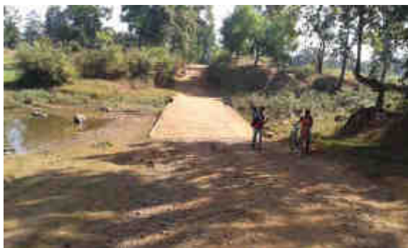
No parapets at low level bridge, Km 8+250
