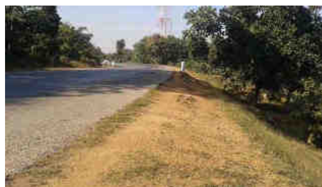
Sharp curve with high embankment without any protection on outer edge, Km 93+600
