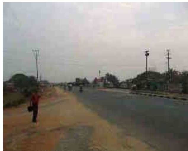
Level difference between side road and main road at Km 251+800
