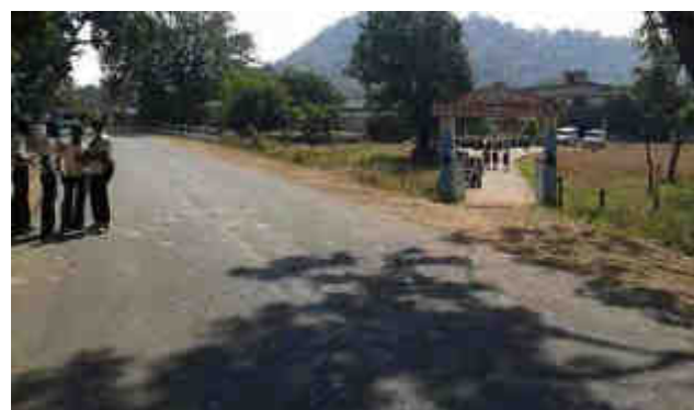
Access road joining SH-15 at skew angle and with steep gradient, Km 24+200
