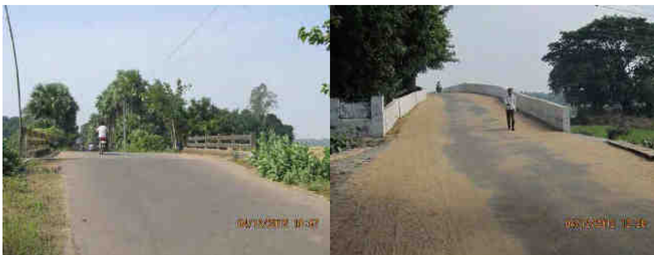
Absence of OHM at Km 24+200 and Km 16+800
