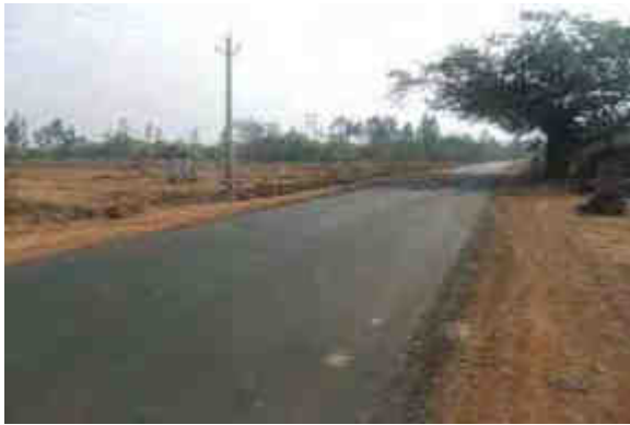
Absence of center line road marking at Km 11+200
