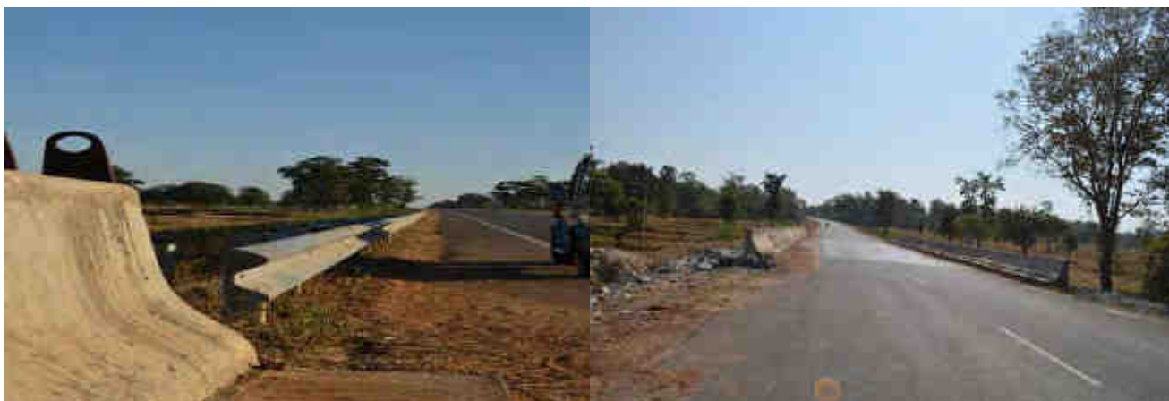
Gap in Crash Barrier and New Jersey Barrier and Absence of OHM on structure
