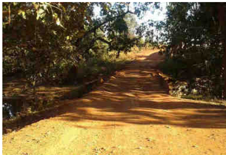
Parapets of culvert not delineate, Km 4+100
