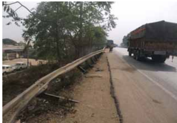
Broken crash barrier at Km 250+300
