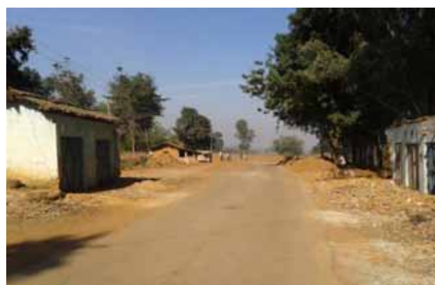
Lack of center line and edge line in the stretch from Km 12+000 to 13+000
