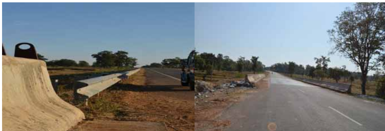
Gap in Crash Barrier and New Jersey Barrier and Absence of OHM on structure
