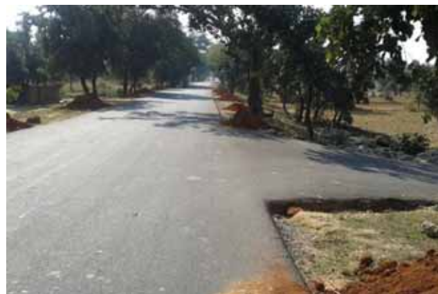
Side road joining with steep gradient, Km 9+000
