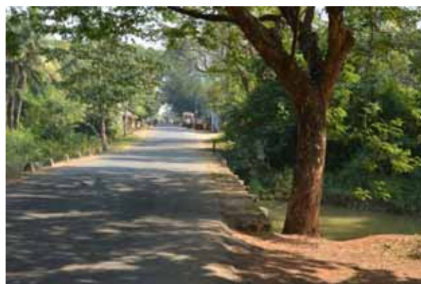
Absence of Parapet wall at Km 41+150
