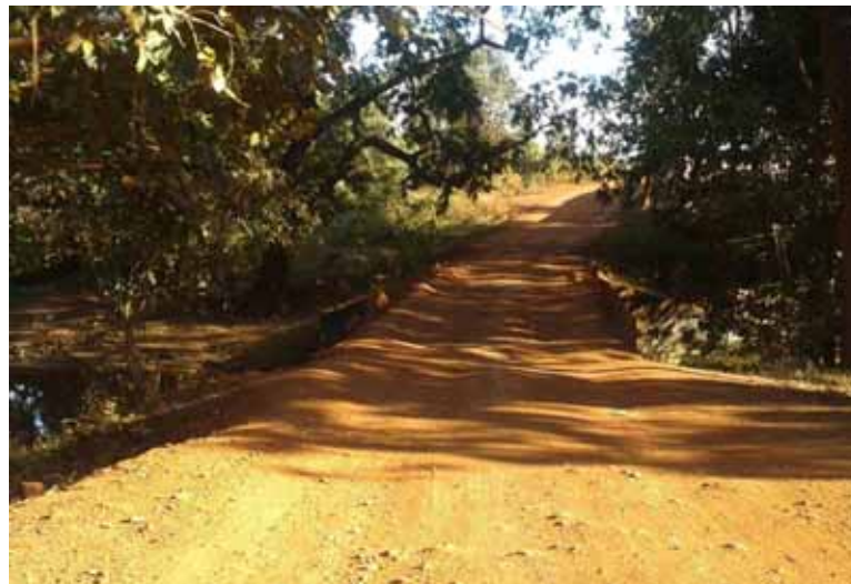
Parapets of culvert not delineate, Km 4+100
