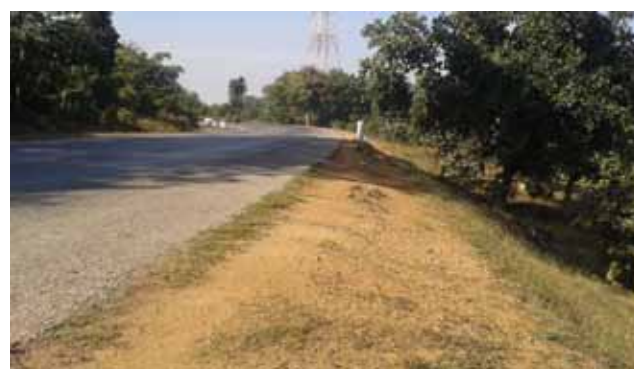
Sharp curve with high embankment without any protection on outer edge, Km 93+600
