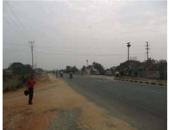
Level difference between side road and main road at Km 251+800
