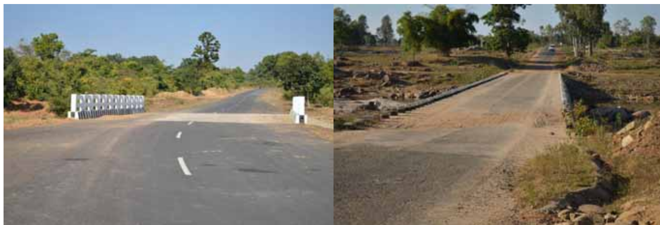
Absence of OHM on structure at Km 44+500 and submersible structure at Km 58+900
