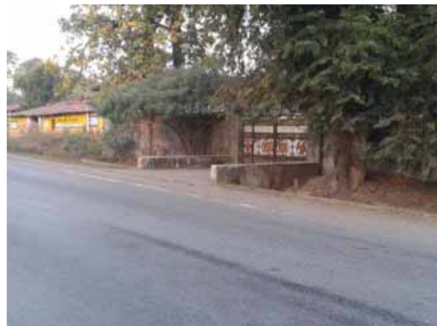
Deep drain and property access very near to the road edge, Km 74+000 to 75+000
