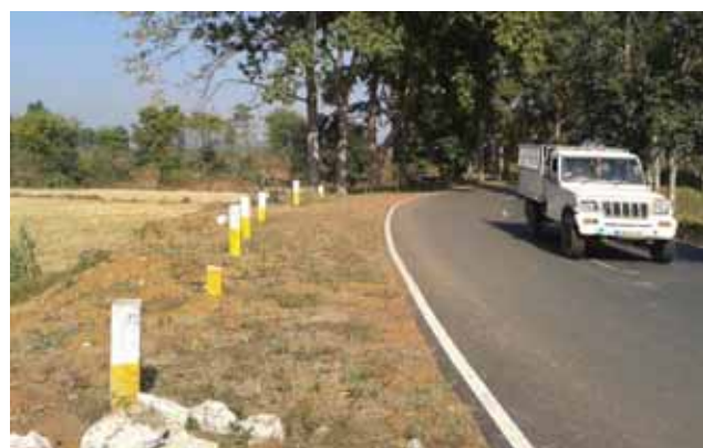
Sharp curve on high embankment without edge protection, Km 9+200
