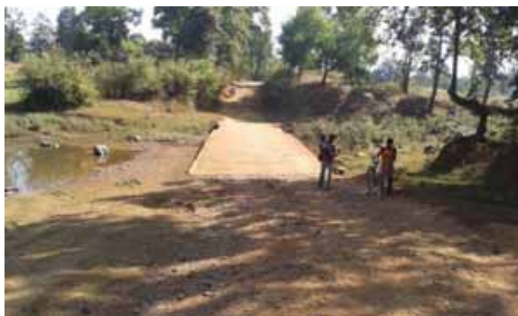
No parapets at low level bridge, Km 8+250
