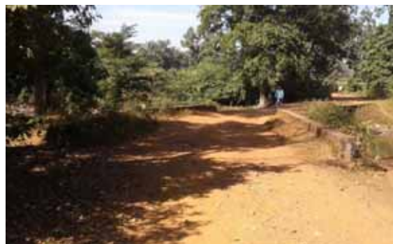
Parapets broken on culvert at Km 11+200
