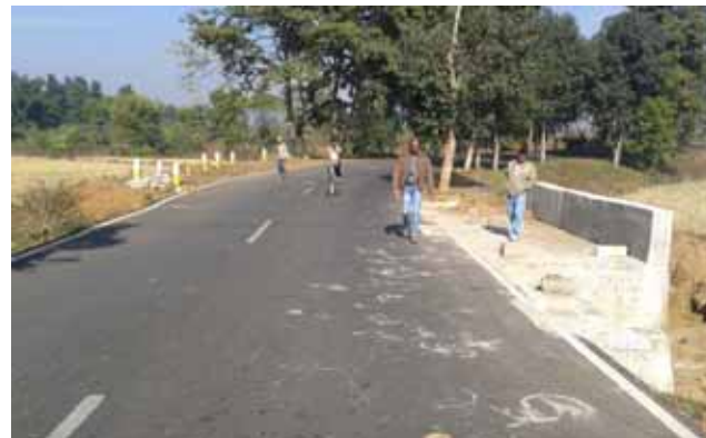
Unprotected approach to culvert under construction – lack of warning signs and barricades, Km 9+200
