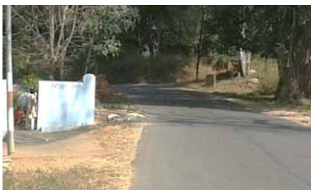
Sharp curve with gradient, side road, and restricted visibility in BUA at Km 16+200
