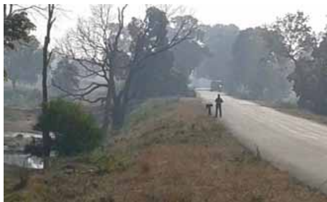
Unprotected approach to bridge with high embankment, Km 6+500
