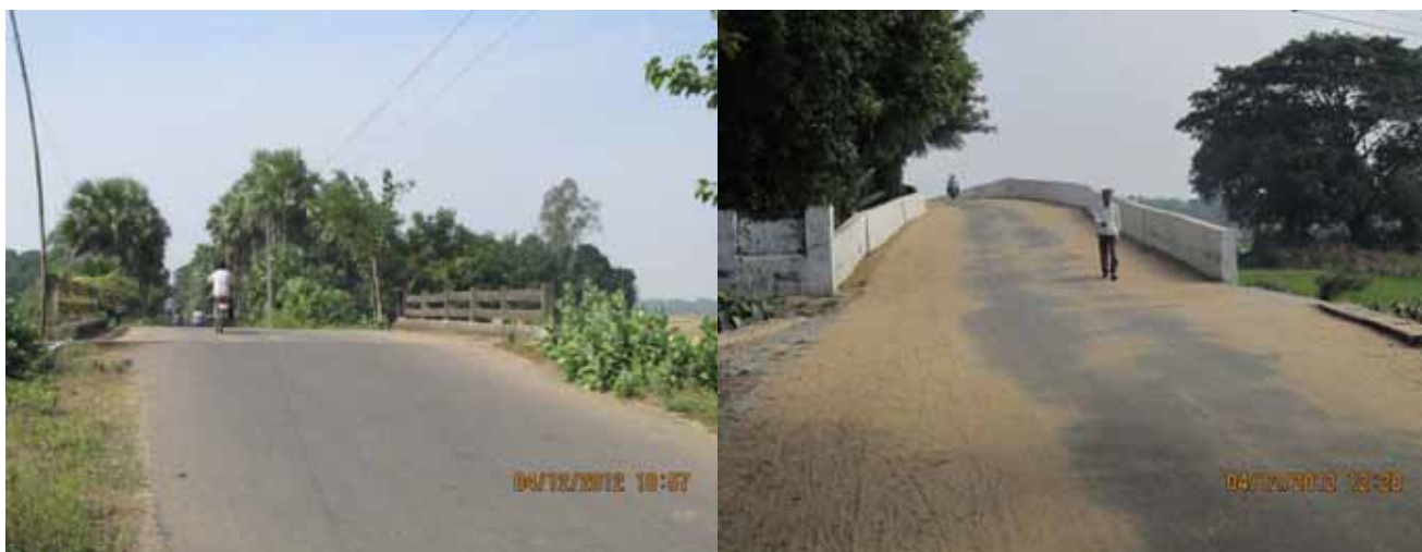
Absence of OHM at Km 24+200 and Km 16+800
