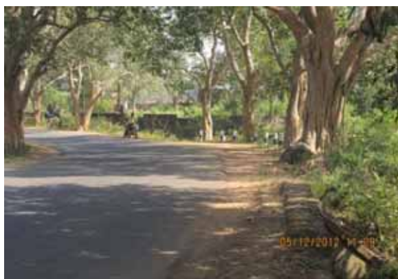
Broken Parapet wall at Km 13+600
