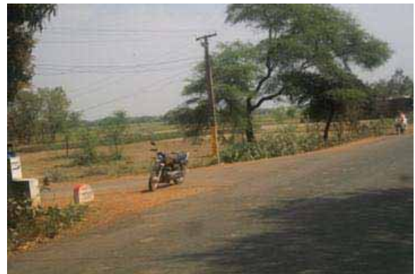
Absence of road marking at Km 35+300
