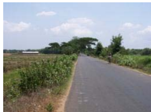
No shoulder and road furniture
