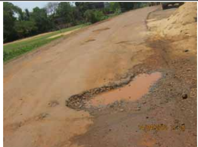
E10: Water logging on damaged road
