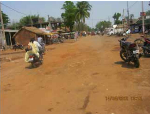
B7: Damaged surface of the road
