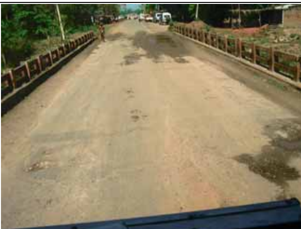
C11: Bad surface of the bridge
