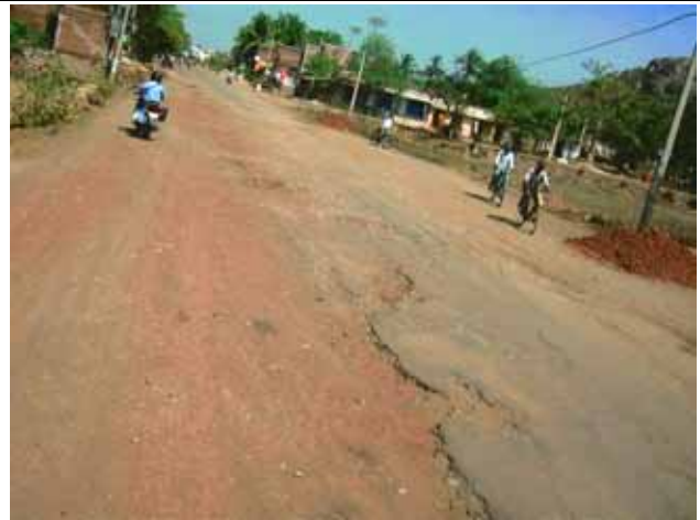
C4: Road in bad condition
