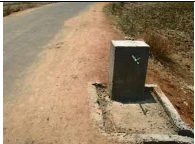
A24: Drinking water source on roadside
