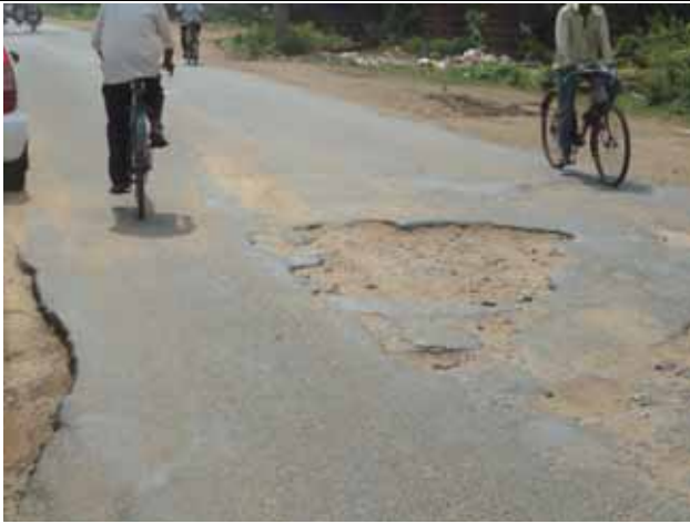
D1: Bumpy road with dangerous edges
