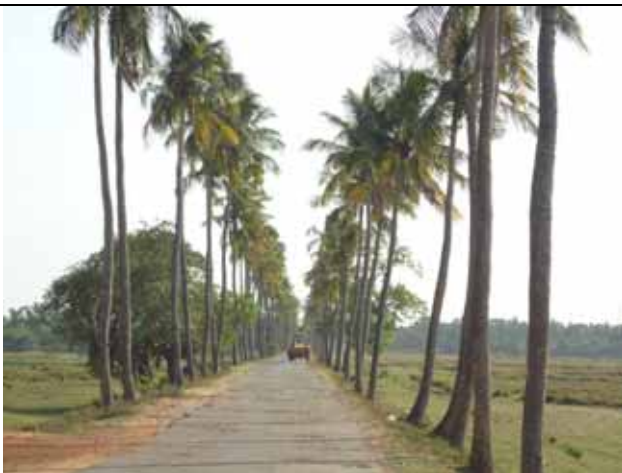
D15: Bad surface of the road
