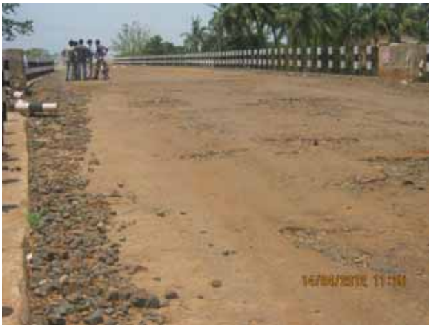
B1: Bad surface of the road
