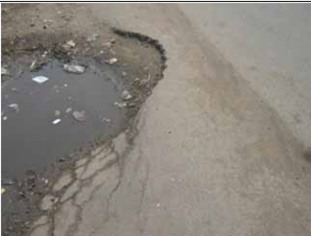
F23: Water logging on road side
