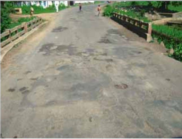
C1: Bad surface of the road
