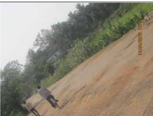
B11: Damaged edges of the road
