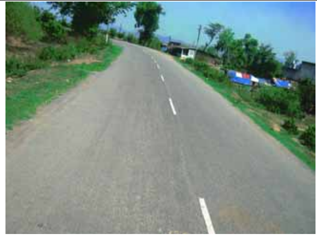
C20: Marking on the road
