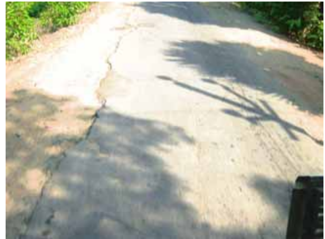
A4: Damaged edges of the road
