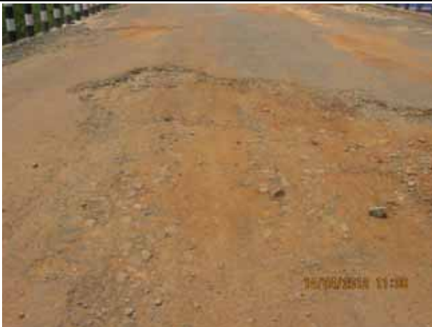
B3: Damaged surface of the road
