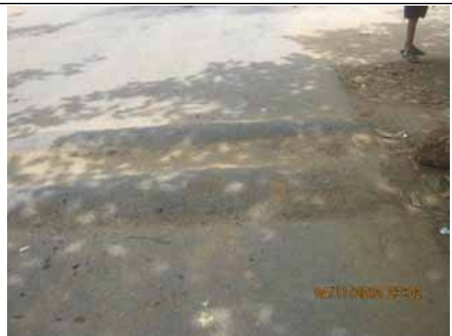
E6: Unmarked speed breakers on the road
