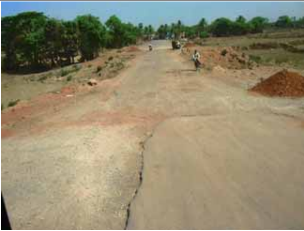
C7: Dangerous edges of the road
