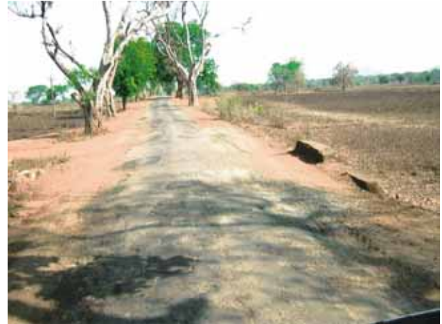
A14: Bad road surface with uneven edges
