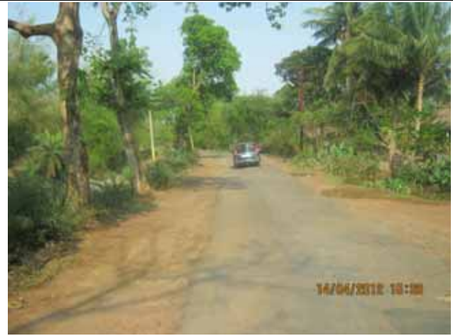
B26: Dangerous edges of the road
