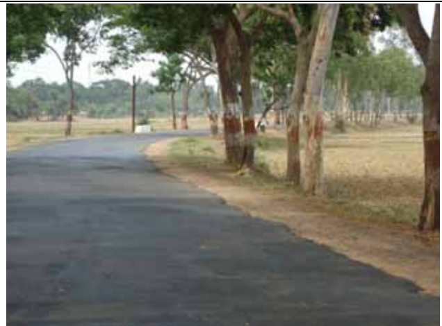
D12: Uneven edges of the road
