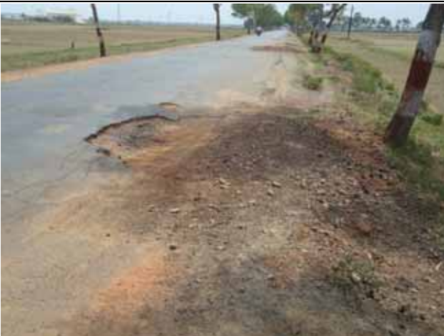
D11: Damaged edges of the road
