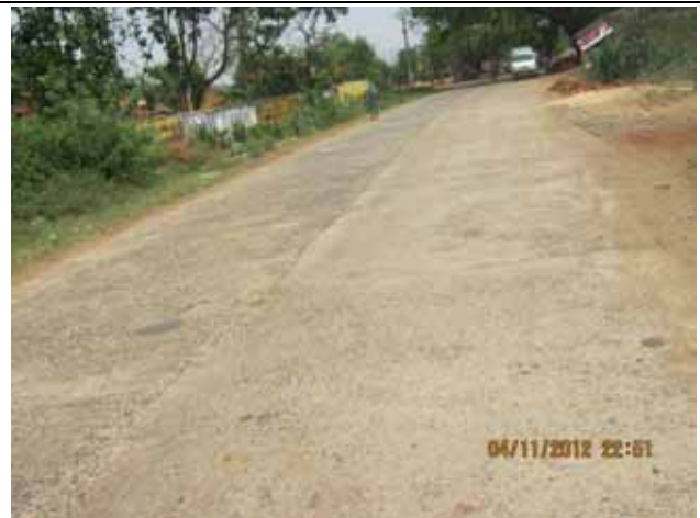
E4: Uneven surface of the road
