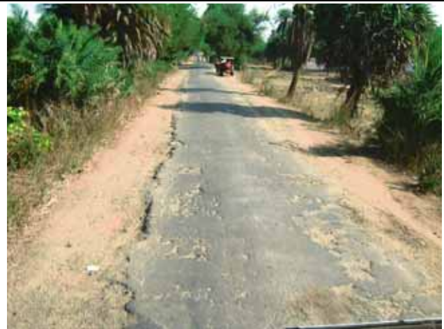
A10: Dangerous edges of the road
