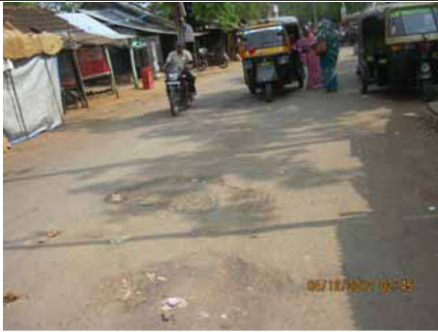
E19: Bad surface of the road
