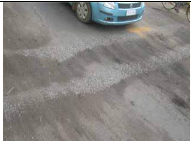
F18: Unmarked speed breaker on the road
