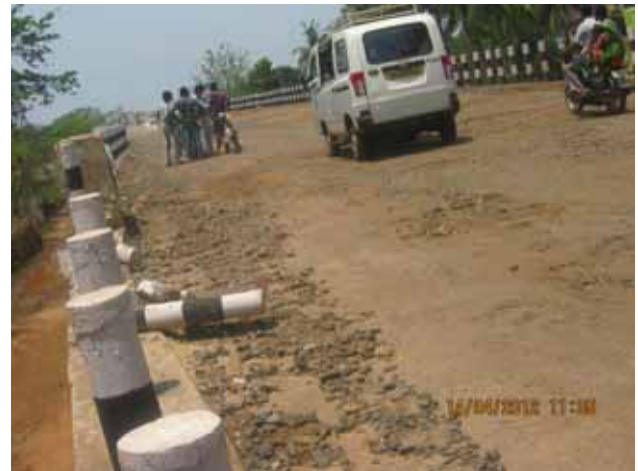
B2: Damaged railing on the bridge
