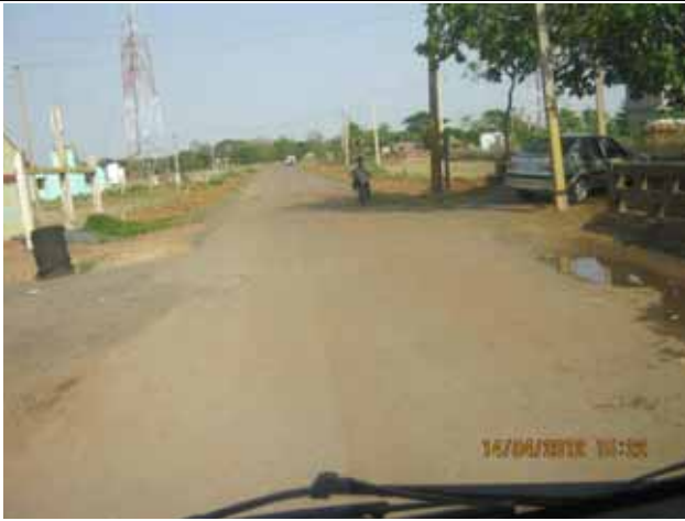
B19: Water logging on the road side
