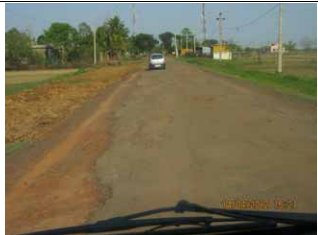
B18: Damaged edges of the road
