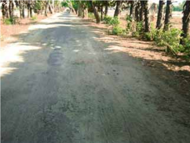
A13: Road in bad condition
