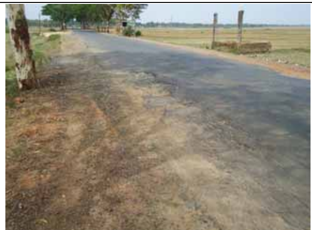
D24: Uneven edges of the road
