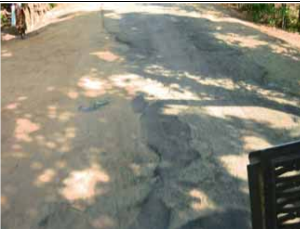
A5: Bad surface of the road
