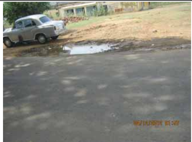
E16: Water logging on road side
