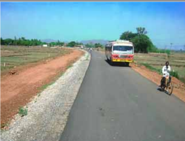
C17: Road with good surface
