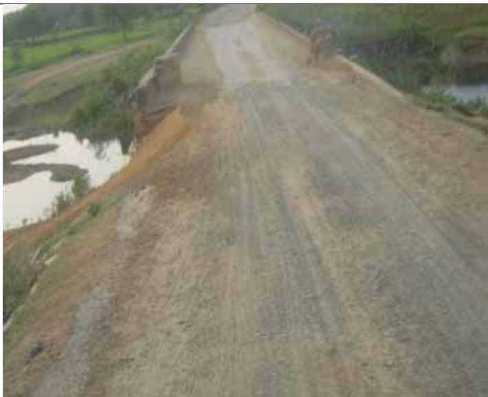
A21: Unsafe joints of road and bridge/culvert
