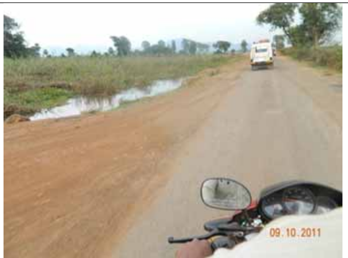
B6: Road widened but culvert work not yet started
