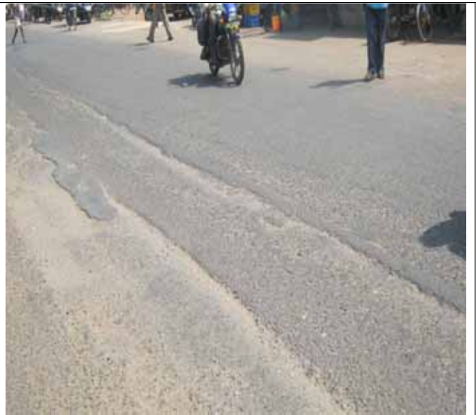
F14: Bad surface of the road
