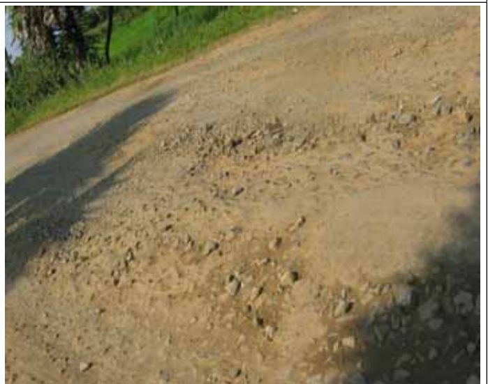
A12: Bad condition of the road
