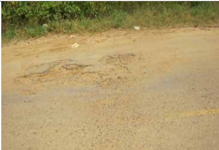
A5: Bad surface of the road
