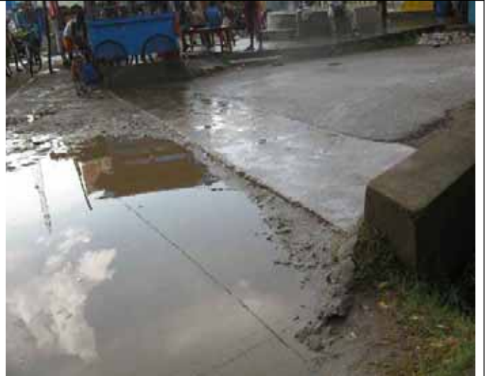
C8: Water logging on road after rain
