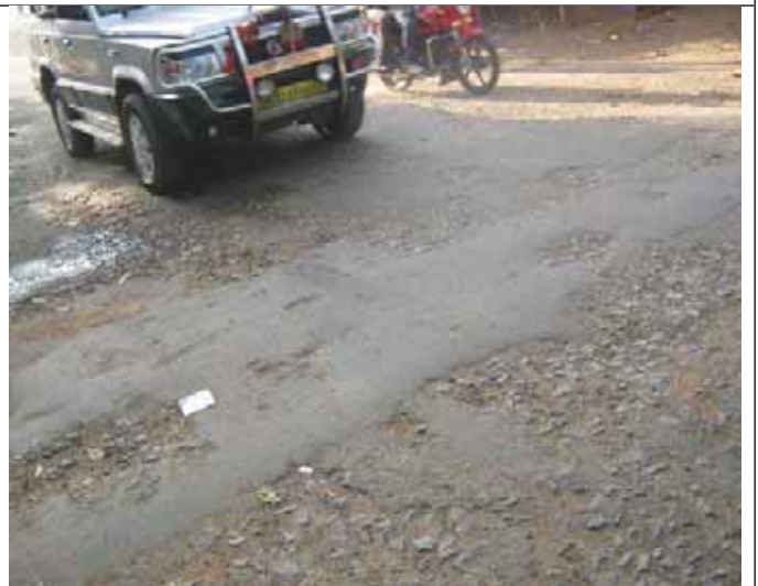
C10: Bad surface of the road
