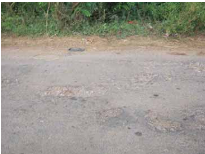
C5: Bad surface of the road
