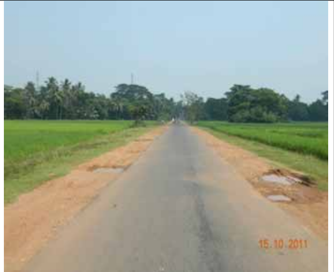
D8: Single lane road, both sides of the road are damaged
