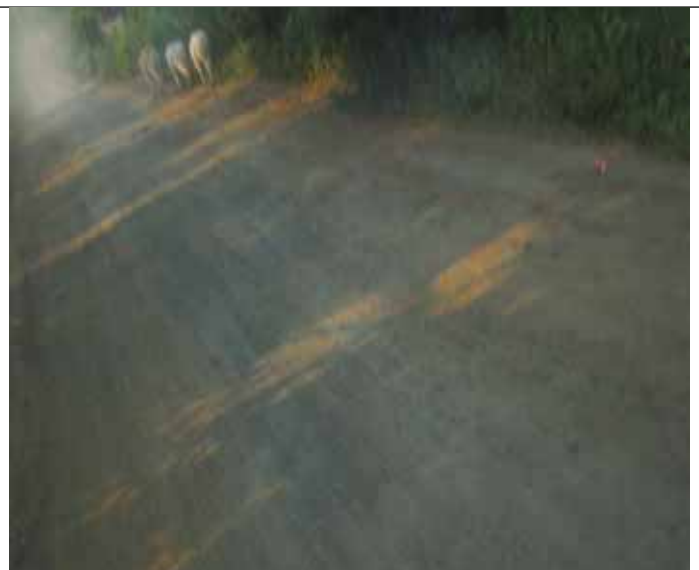
A18: Single lane road with damaged edges
