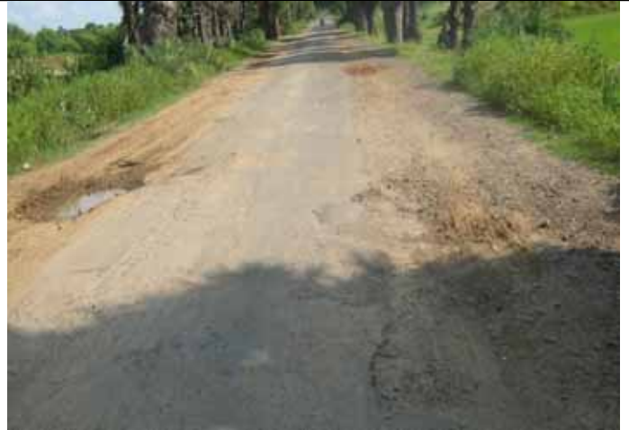
A14: Single lane road with damaged edges
