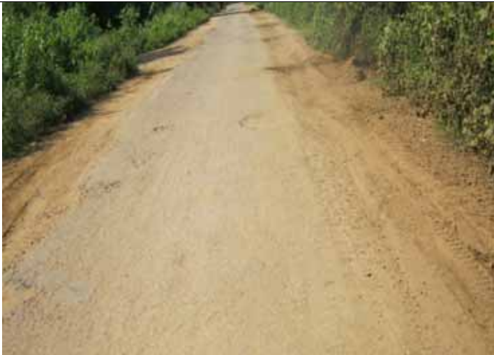
A3: Single lane road with bad surface
