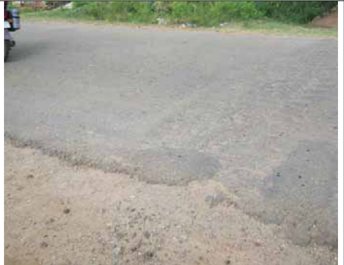
C4: Damaged edges of the road
