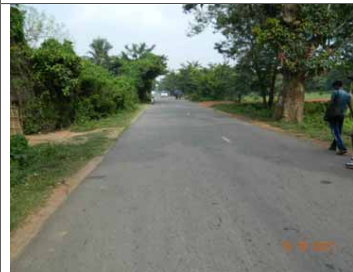
D15: Road marking is not clearly visible
