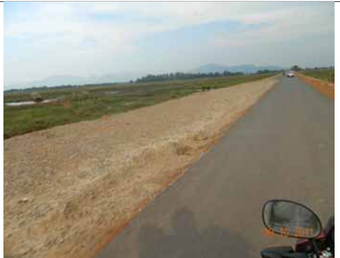
B4: One lane of the road is complete other is under process
