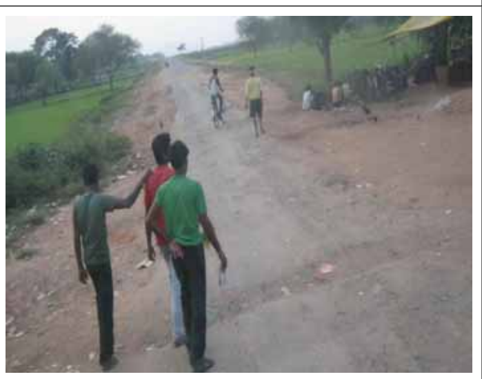
A24: Single lane road in bad condition
