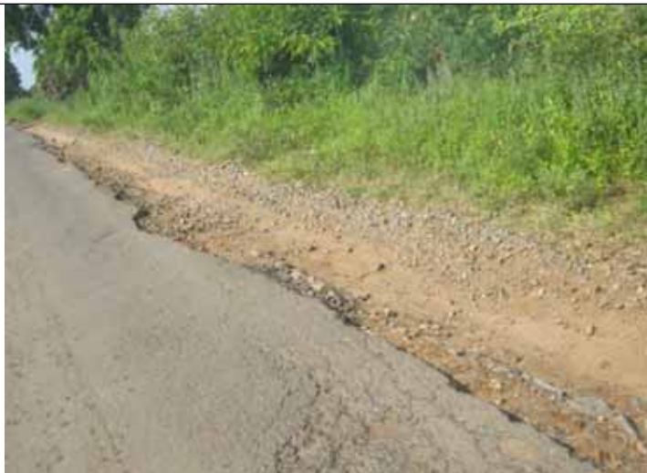
A9: Damaged edges of the road
