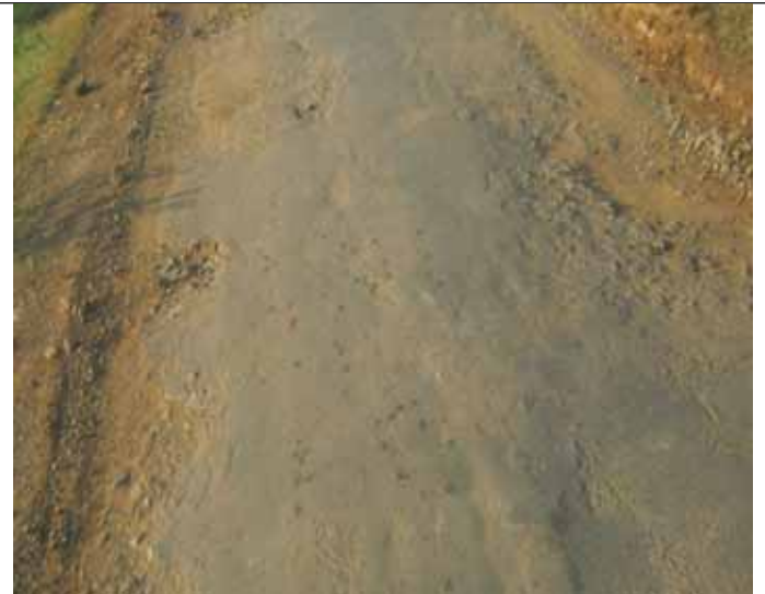
A16: Single lane road in bad condition
