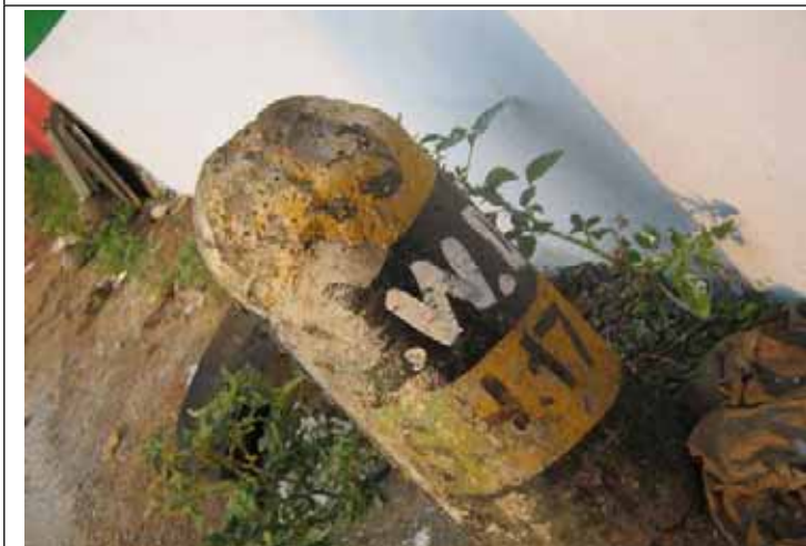
C17: Road information pillar
