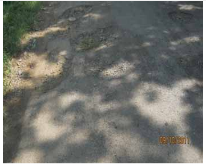
E10: Bad surface of the road
