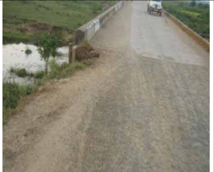
A20: Unsafe joints of road and bridge/culvert
