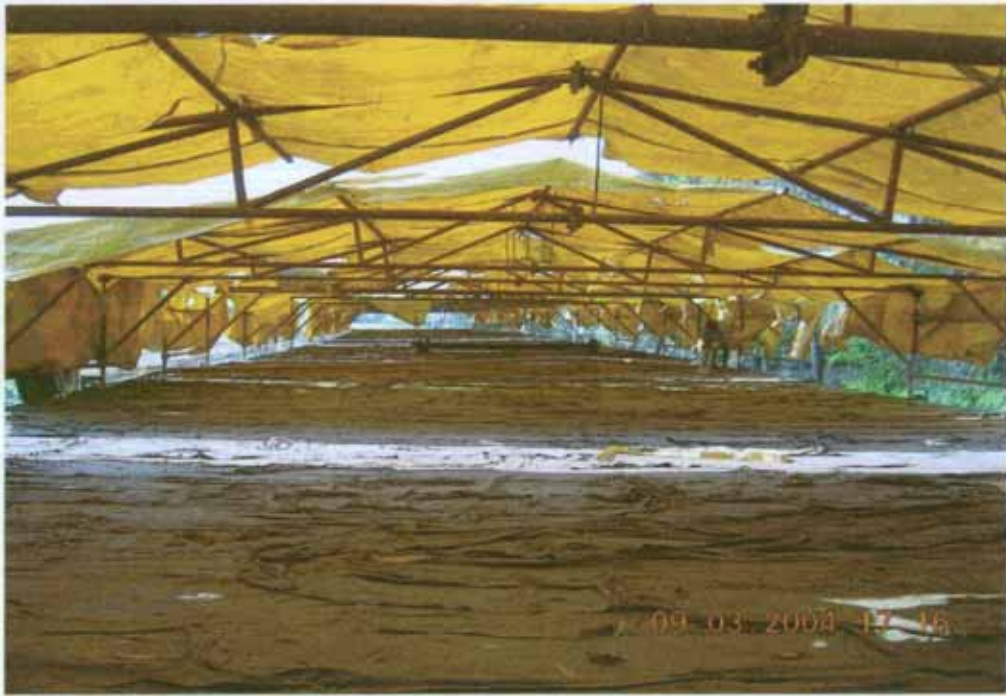
Protection of pavement using a movable tent & Curing with Wet Hessian Cloths
