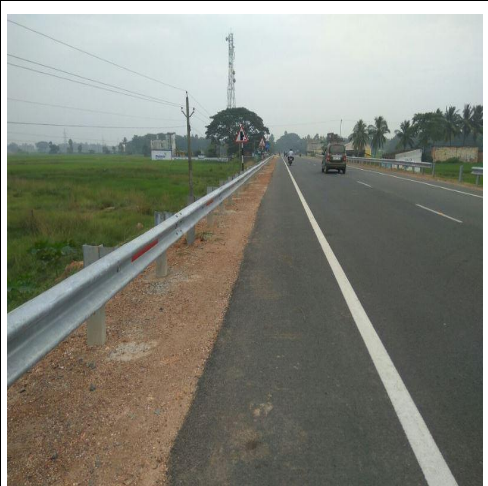
Metal Beam Crash Barrier at 34+794 to 34+850 LHS
