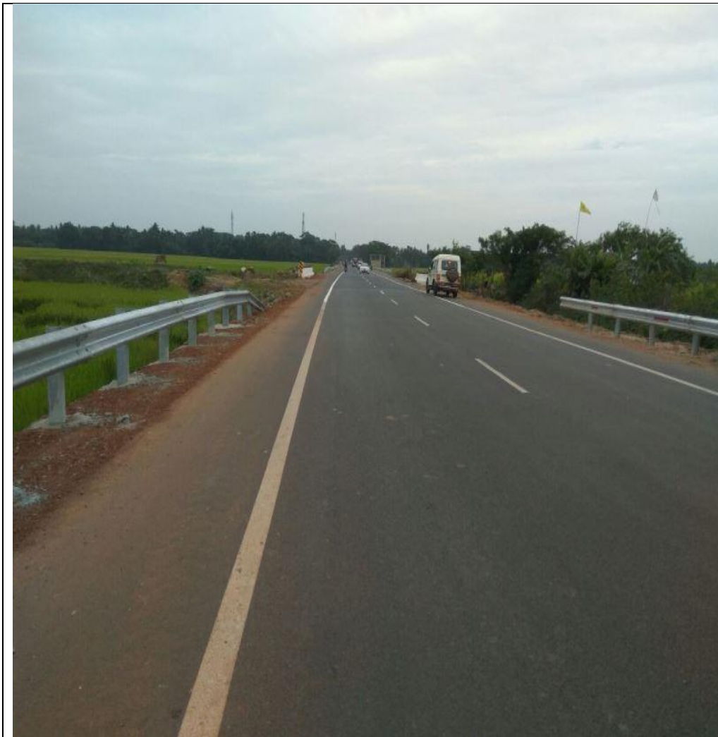
Metal Beam Crash Barrier at 31+414 to 31+670 LHS
